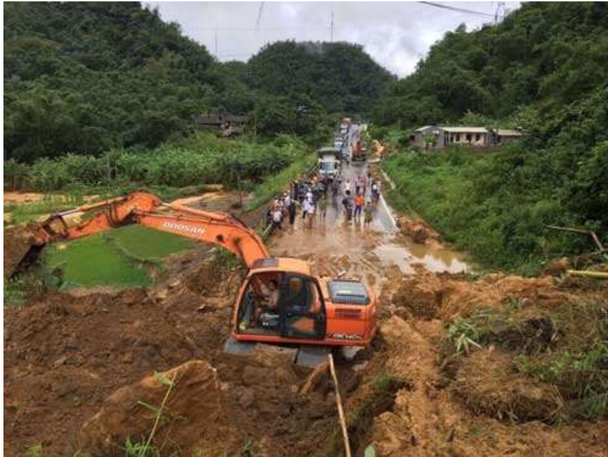
Landslide in Dong Bang commune, Mai Chau, Hoa Binh, 14/8/16
