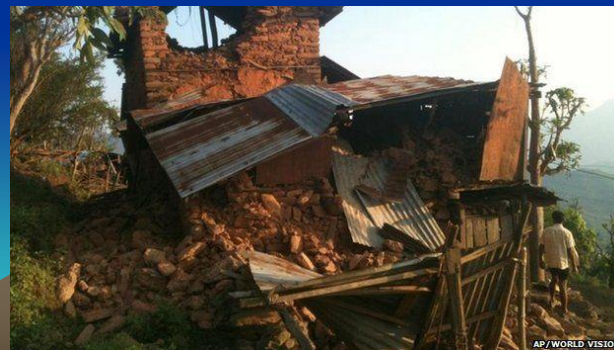
(7) Damaged Animal Shelter
