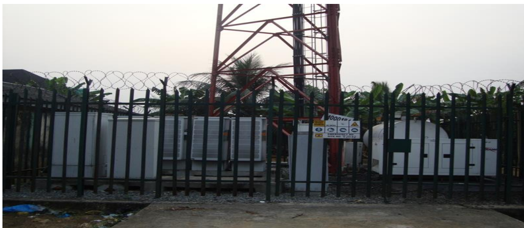
Fig 1.2: A Typical GSM Telecommunication Mast Facility (Source: Hart L. & Jackson K.P, 2006)
