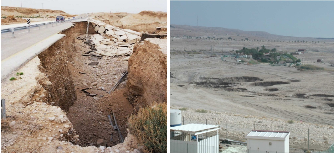
Figure 1. left) Influence of gully incision processes on infrastructure, right) sinkhole field near a beach resort.
