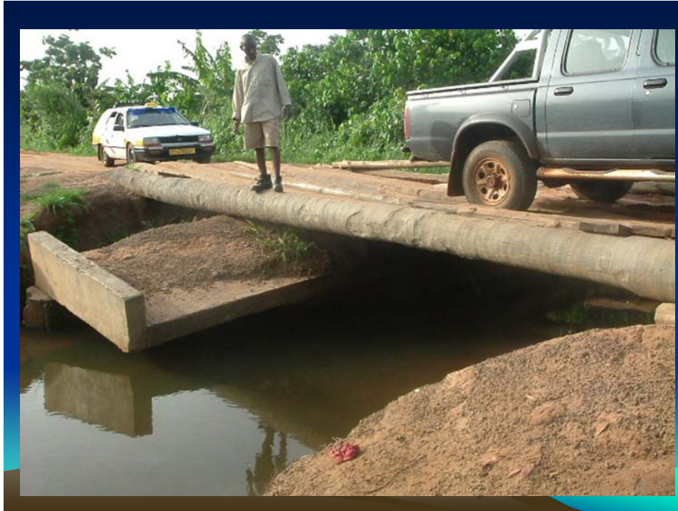
Fig 5: Accessing broken culvert on the road
