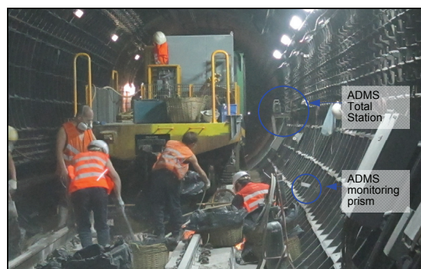
Figure 19. ADMS prisms may be disturbed by others in tunnel.
