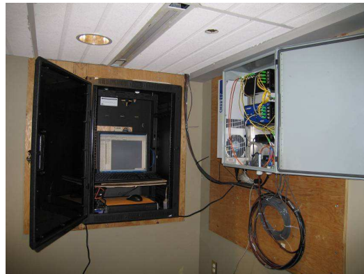
Figure 16 - Central Measurement Point with dedicated PC (left) and Fiber Optic reading unit with switch (right)
