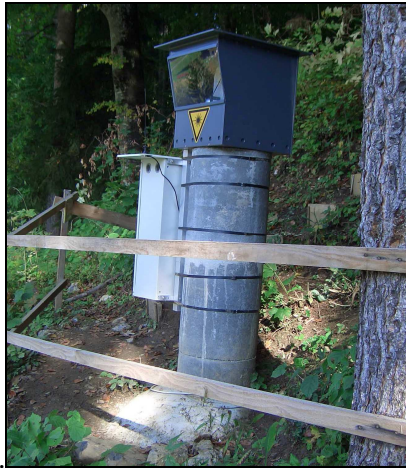
Figure 8 - ROBOVEC installed on a pillar
