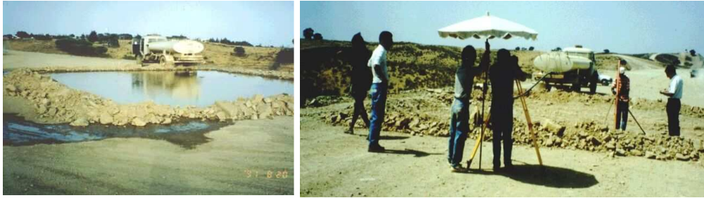
Figure 10 – Fill of VLA. Collapse test
