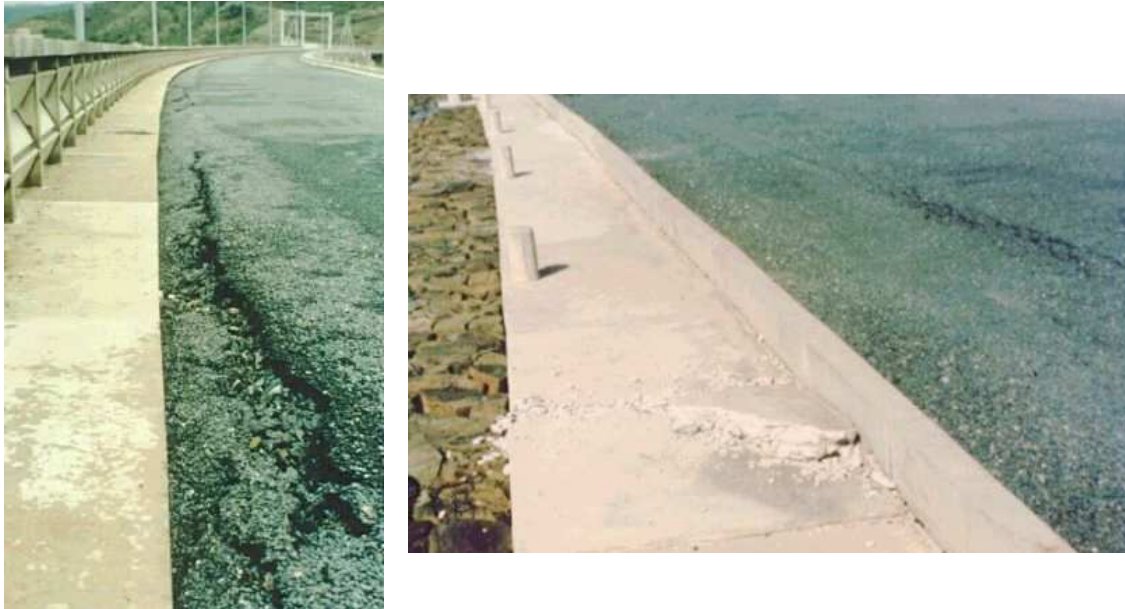
Figure 8 – Beliche Dam. Aspects of anomalies detected at the crest
