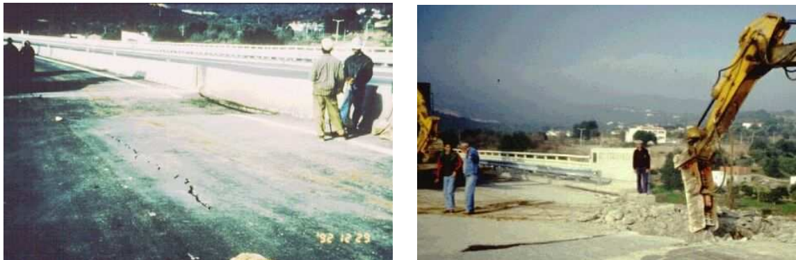
Figure 11 – Fills close to Rio Seco Bridge. Excessive settlements, cracking and rehabilitation works
