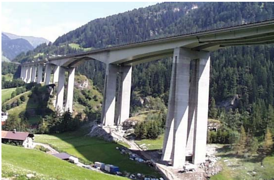
Fig. 7: View of the Colle Isarco Bridge on the Brennero Highway in Italy
