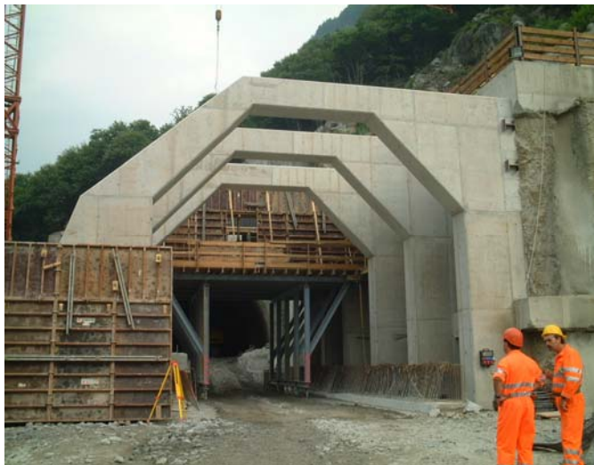
Figure 9: Support Buttresses at the south portal of the new Alptransit Gotthard tunnel
